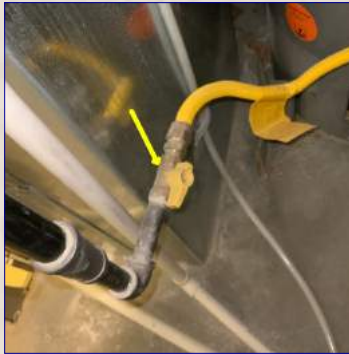
The Water Heater gas shut off valve.
