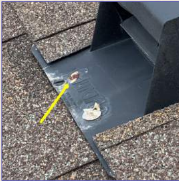
There are exposed nail heads securing the flashing to the roof. Exposed nail heads can allow water to penetrate the roof. Recommend a licensed roofer to seal the nail heads.
