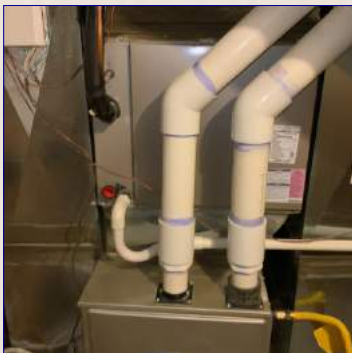
The evaporator coil cabinet.
