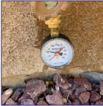
The water pressure at the hose bib.
