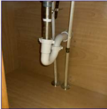
The bathroom plumbing view.
