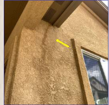
The stucco siding had moisture staining. Recommend a licensed contractor evaluate and repair as needed.
