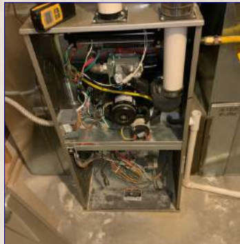
The furnace view, cover off
