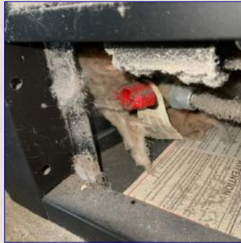
The fireplace gas shut off valve.
