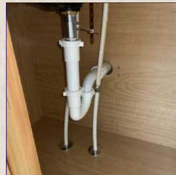
The bathroom plumbing view.
