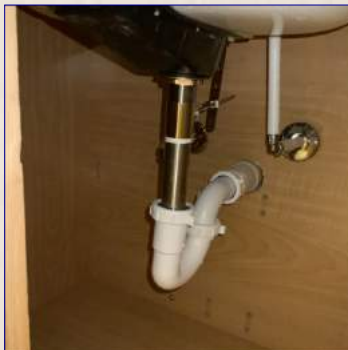
The bathroom plumbing view.
