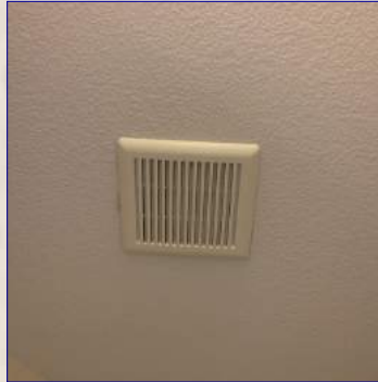
The exhaust fan operating.
