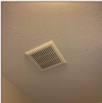
The exhaust fan operating.
