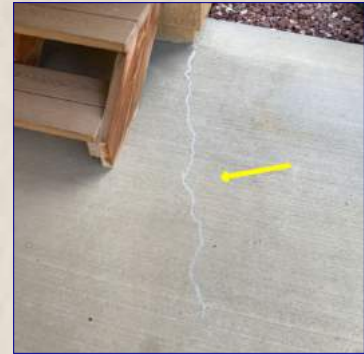
The patio has typical cracks. Recommend a professional contractor seal the cracks to help protect the cement from damage.
