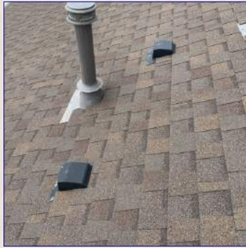
The Bathroom Vent(s)
