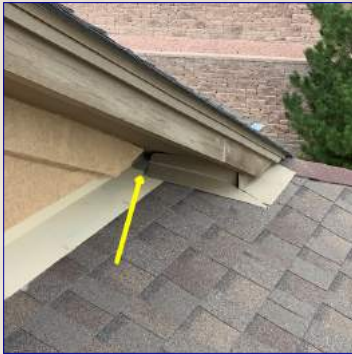
There were gaps at the flashing. Recommend a licensed roofer evaluate repair as needed.
