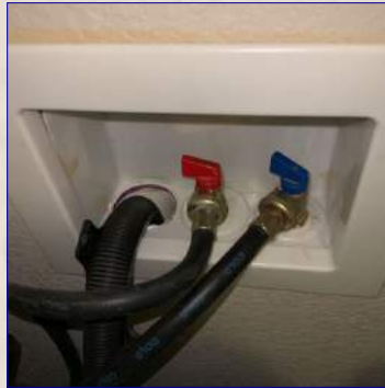
Laundry, washer hook-up view
