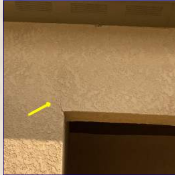
The stucco siding had typical cracking present in one or more areas. Monitor and repair as needed.
