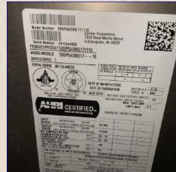
The furnace, data tag
