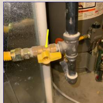
The gas shutoff valve.
