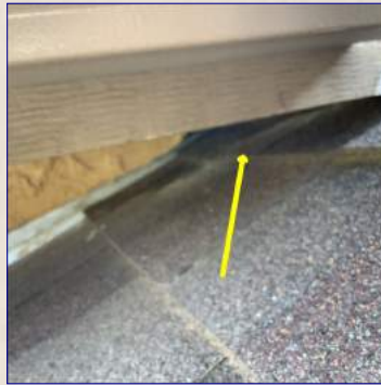
There were areas of missing flashing. Recommend a licensed roofer install flashing.
