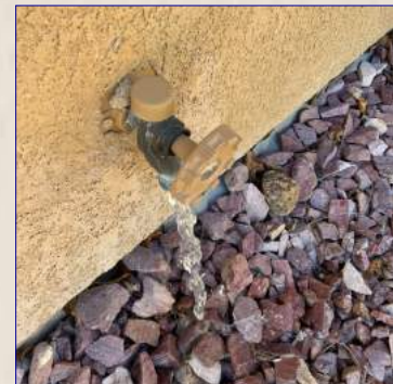
Hose bib operational.
