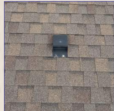
The Bathroom Vent(s)
