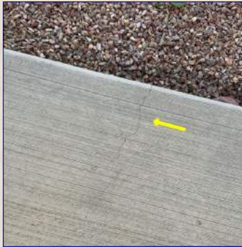
The patio has typical cracks. Recommend a professional contractor seal the cracks to help protect the cement from damage.
