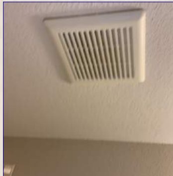
The exhaust fan operating.
