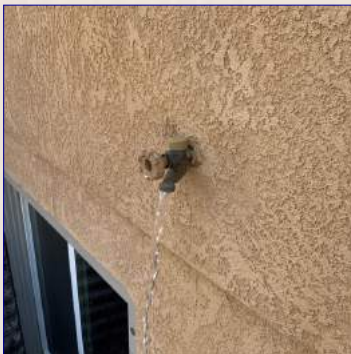
Hose bib operational.
