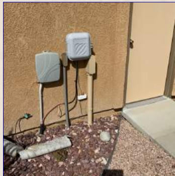
The electrical service entrance.
