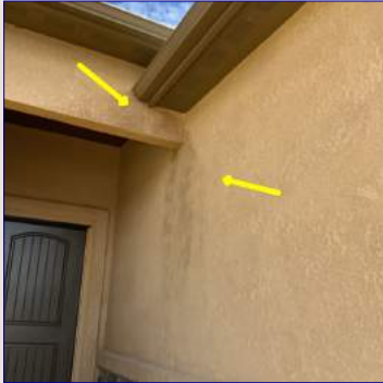
The stucco had moisture staining. Recommend a licensed contractor evaluate and repair as needed.
