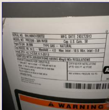
The Water Heater Data Tag
