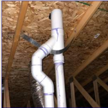
Hvac plumbing view
