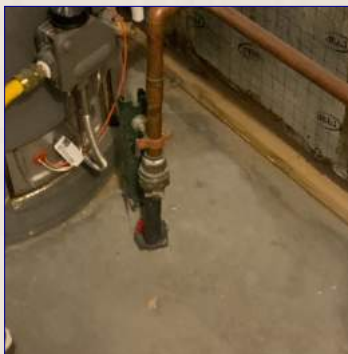
The water entry piping.
