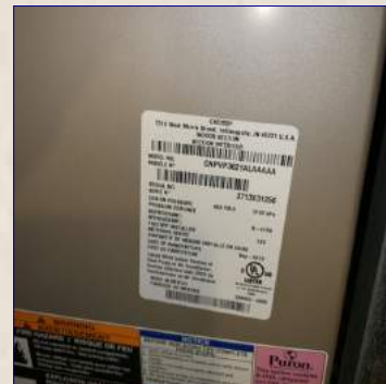
The air conditioner coils data plate.
