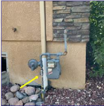
The main gas shutoff valve.
