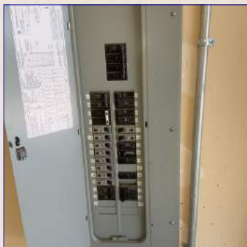
The main electrical service panel.
