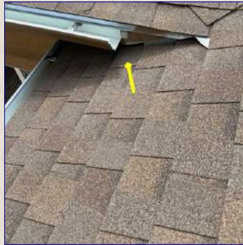
The fascia needs routine painting maintenance. Recommend a professional painter repair/paint the fascia.
