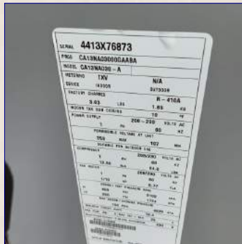
The air conditioner compressor/condenser data plate.
