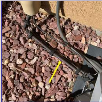
There is damaged and/or missing insulation on the air conditioner refrigerant line. Recommend replacing insulation.
