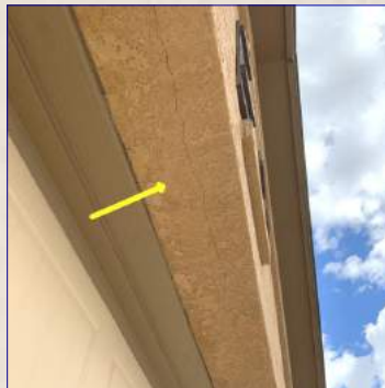
The stucco siding had typical cracking present in one or more areas. Monitor and repair as needed.
