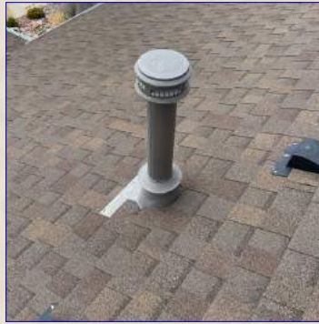
The HVAC Vent(s)
