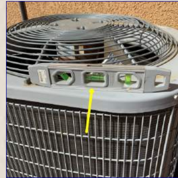
The air conditioner condensing unit is not level. Recommend a professional contractor to re-level the unit.
