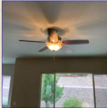
Ceiling fan operating
