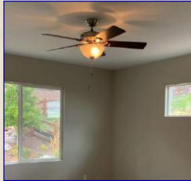
Ceiling fan operating
