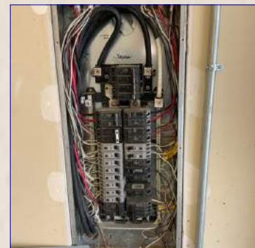
The main electrical service panel-cover removed.
