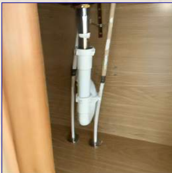
The bathroom plumbing view.
