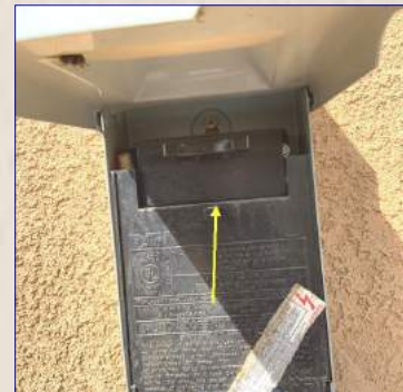
The air conditioner compressor/condenser electrical shut off switch.
