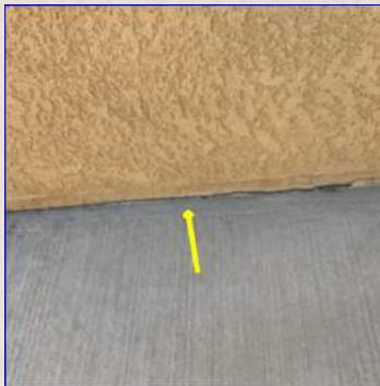
There is a gap between the patio and the house. Recommend sealing the gap between the patio and the house to help prevent water penetration.
