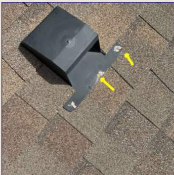
There are exposed nail heads securing the flashing to the roof. Exposed nail heads can allow water to penetrate the roof. Recommend a licensed roofer to seal the nail heads.
