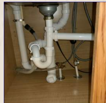
Kitchen plumbing view
