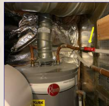
The Water Heater water shut off valve.
