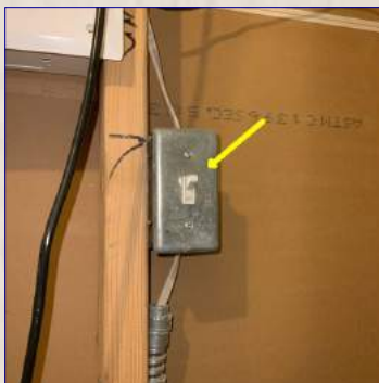
The electrical shutoff switch.
