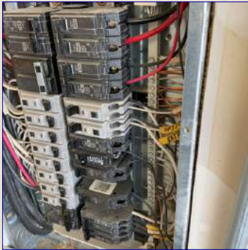
The main electrical service panel-cover removed.
