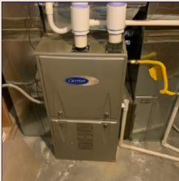
The furnace area
