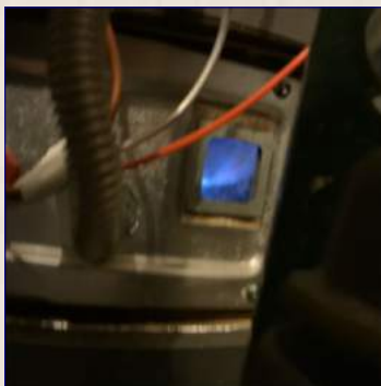
The water heater operating.
